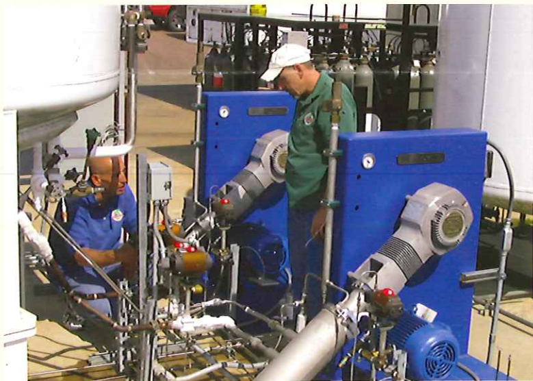
Bud Klotz, vice president (left) and Mark Daniels, west coast sales engineer, install a remote pump station for a distributor's end-user customer.
